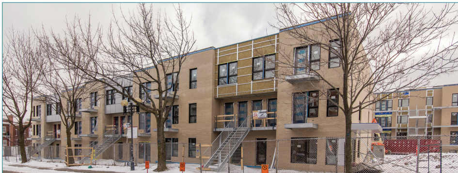
The Petits et grands Housing Co-operative, a project of 46 dwellings for families, in construction in Hochelaga-Maisonneuve district.
